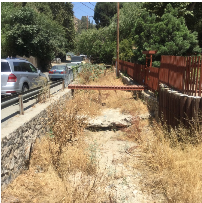
Looking upstream at Kagel Canyon channel and Str. 7 from Str. 6 (East Trl)
